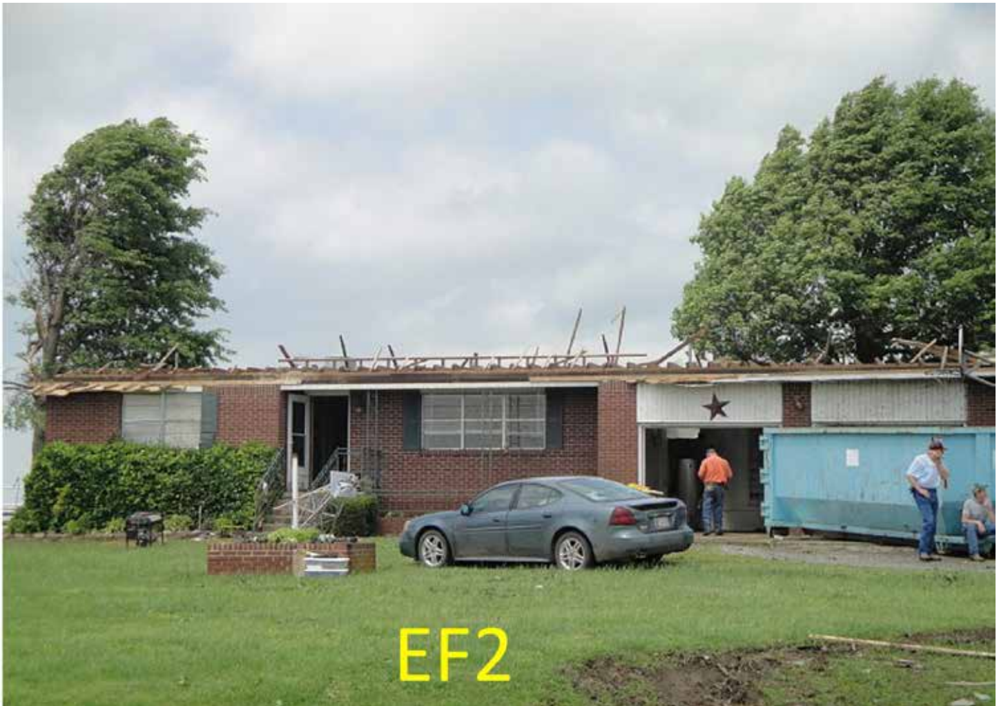
Figure 6.85f. Roof damage from an EF2 tornado on May 7, 2012 near Tulsa, Oklahoma (Source/Credit: http://www.srh.noaa.gov/tsa/?n=weather-event_2012aprfflood ).
