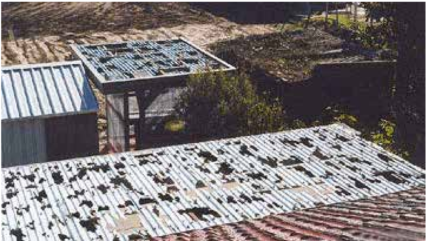
Figure 4.74c. Hail damage to corrugated plastic shelters, mid-western United States (Source/Credit: NWS).
